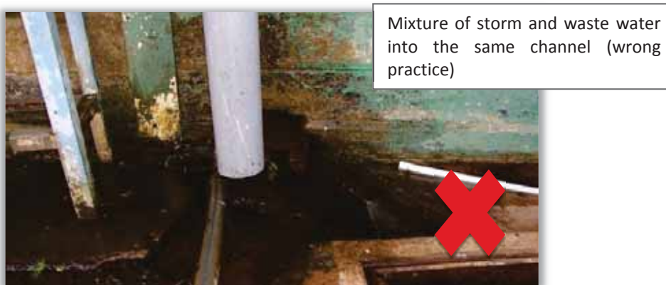
Figure 12: Bad practice in waste water treatment
